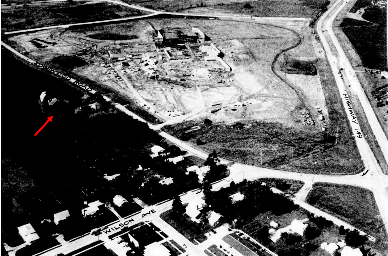
Viewed from the northeast, the mall begins to take shape across Edgewood Road from the east homestead site. Cedar Rapids Gazette, July 23, 1978
